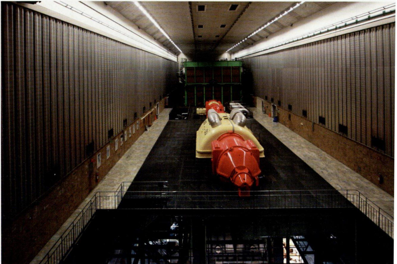
No 2 turbine hall at the Stenungsund power station in Sweden. One of the older 160MW generators is seen. Photo Lars Hansson
